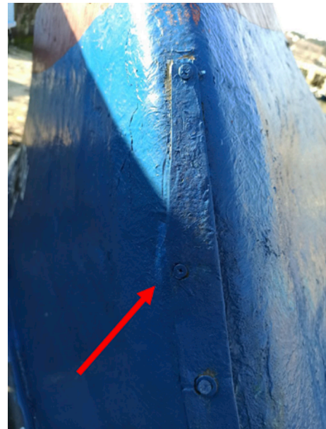
Fig. 34. Application of the bolted joining method in joining steel to the wooden part of the bow.
